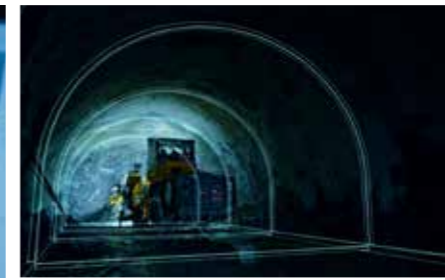
When using the drill plan generator you will download the 3D model of the tunnel into the drill rig.
