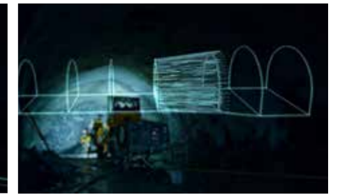
When generating the drill plan the exact location of the drill rig and the planned shape of the tunnel will be taken into consideration.
